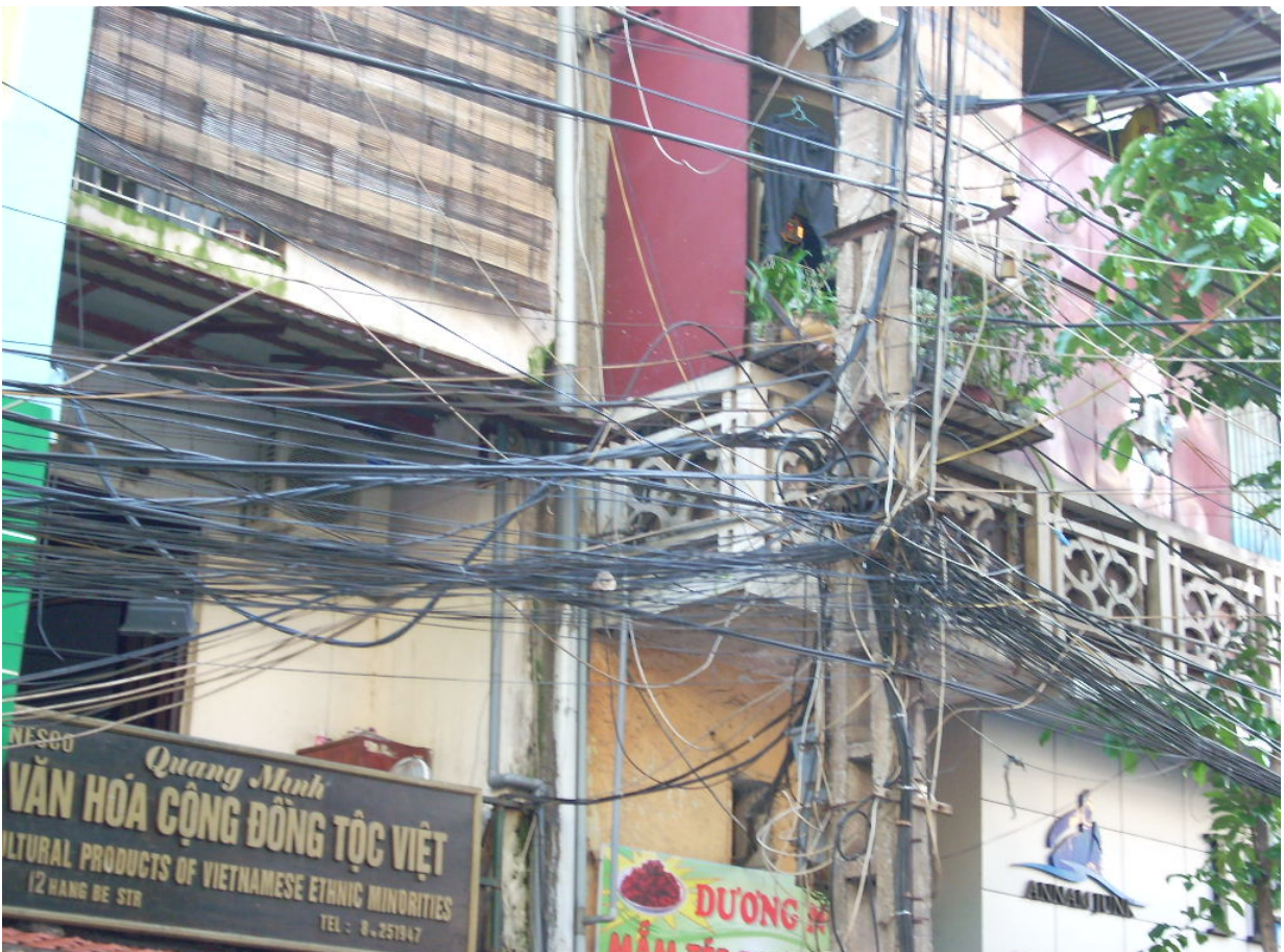
A common electric circuit in the Hanoi's streets (photo taken by the Greek Delegation to the 39 th International
